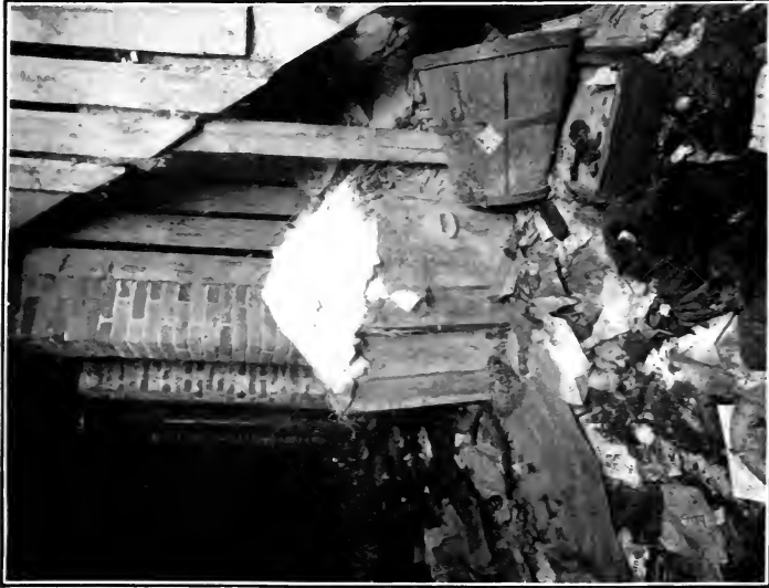
Cellar rendered filthy by mixture of garbage and ashes.
