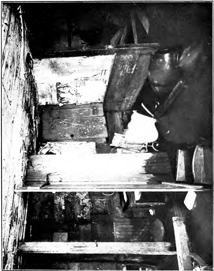
Cellar toilet used by 3 families. Only approach to toilet is over piece of joist shown in picture. 12 inches of water in cellar when picture was taken.
