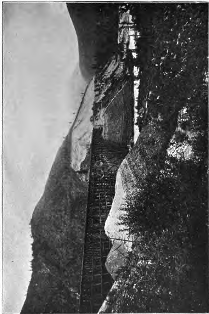
FIG. 50.—HYDRAULIC FILLS, PARTIALLY COMPLETED, AT MOUNTAIN CREEK, B. C., CANADIAN PACIFIC RAILWAY.
