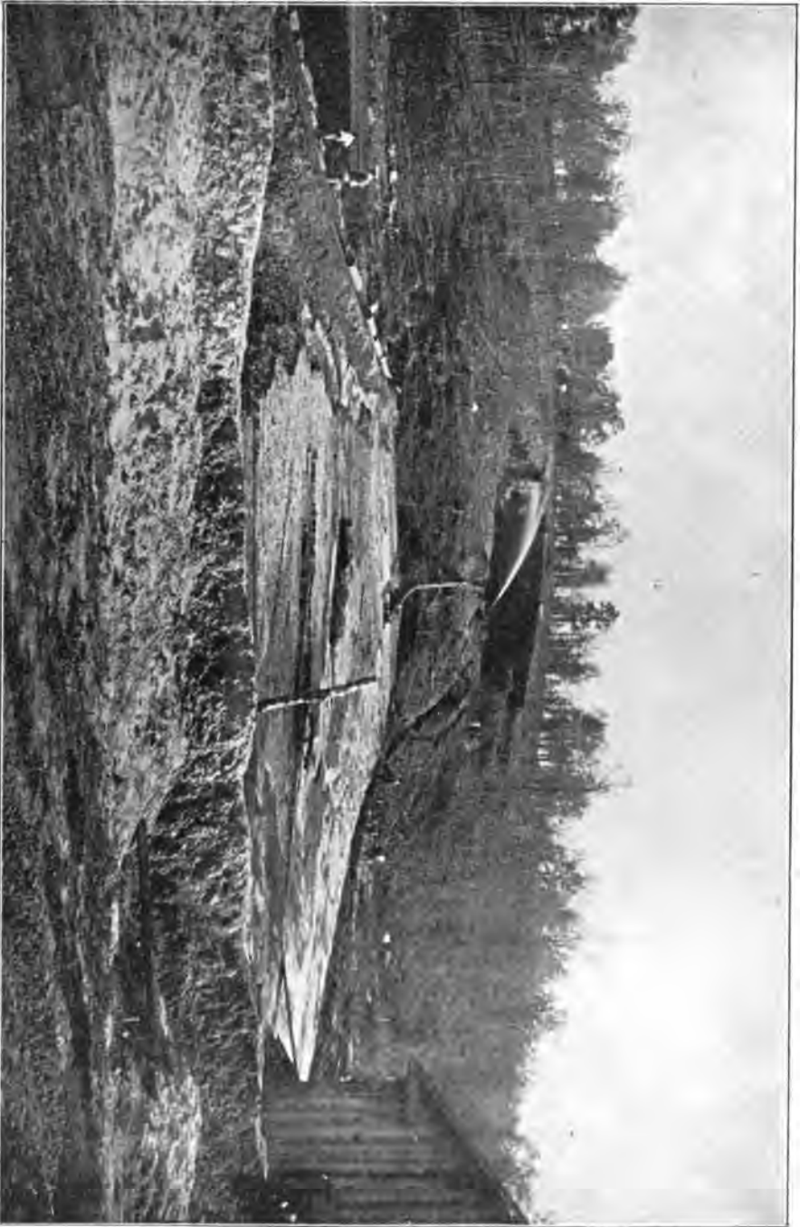
FIG. 42.—HYDRAULIC-FILL DAM, AT TYLER, TEXAS, IN PROCESS OF CONSTRUCTION. Water supplied by pump in building at right of picture.
