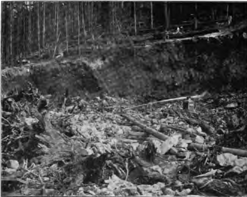
FIG 54.—NORTHERN PACIFIC RAILWAY, HYDRAULIC-FILL CONSTRUCTION. VIEW IN PIT SHOWING HYDRAULIC GIANT IN ACTION.
