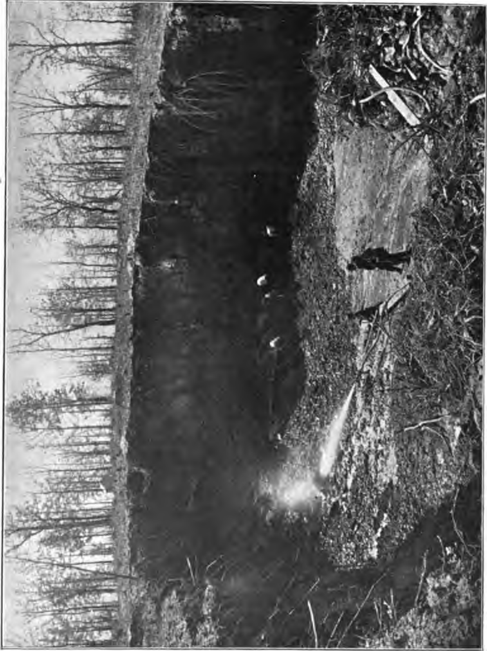
FIG. 41.—HYDRAULIC SLUICING FOR BUILDING DAM AT TYLER, TEXAS. The small stream here shown did the entire work.
