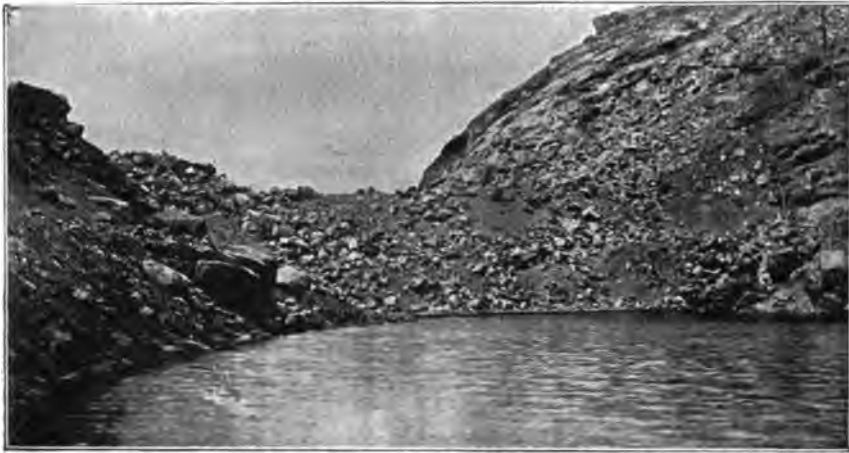
FIG. 19.—MORENA ROCK-FILL DAM IN PROCESS OF CONSTRUCTION. SHOWING TOP OF TOE-WALL ABOVE THE WATER-LINE.
