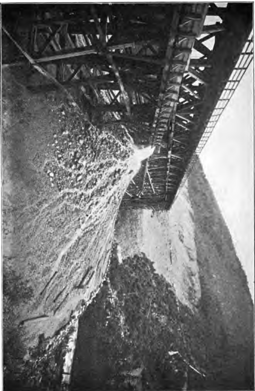
FIG. 51.—HYDRAULIC FILLING OF HIGH TRESTLE AT MOUNTAIN CREEK, B. C., ON CANADIAN PACIFIC RAILWAY, NEAR VIEW OF DUMP.
