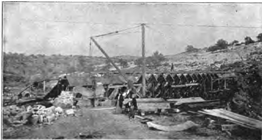
FIG. 112.—ASH FORK, ARIZONA, STEEL DAM, VIEW OF STEEL CONSTRUCTION FROM LOWER SIDE.
