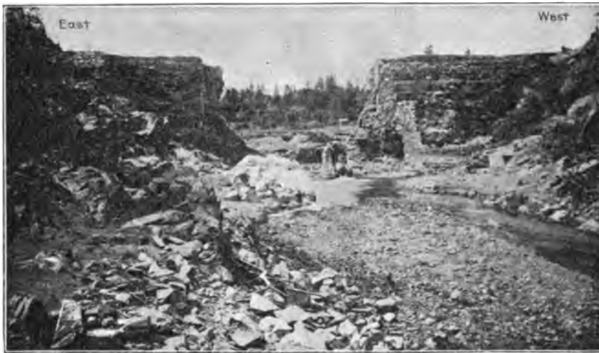
FIG. 117.—LYNX CREEK DAM, ARIZONA, AFTER RUPTURE BY FLOOD. VIEW FROM BELOW.
