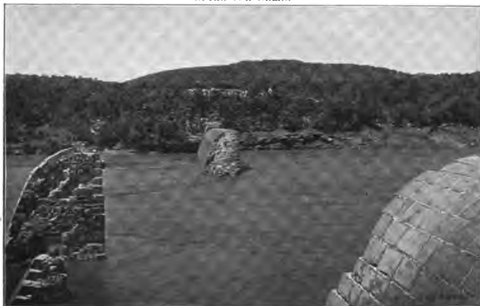
FIG. 123c. —AUSTIN DAM, TEXAS, AFTER SUBSIDENCE OF FLOOD OF APRIL 7, 1900. Showing section of masonry moved bodily down-stream.
