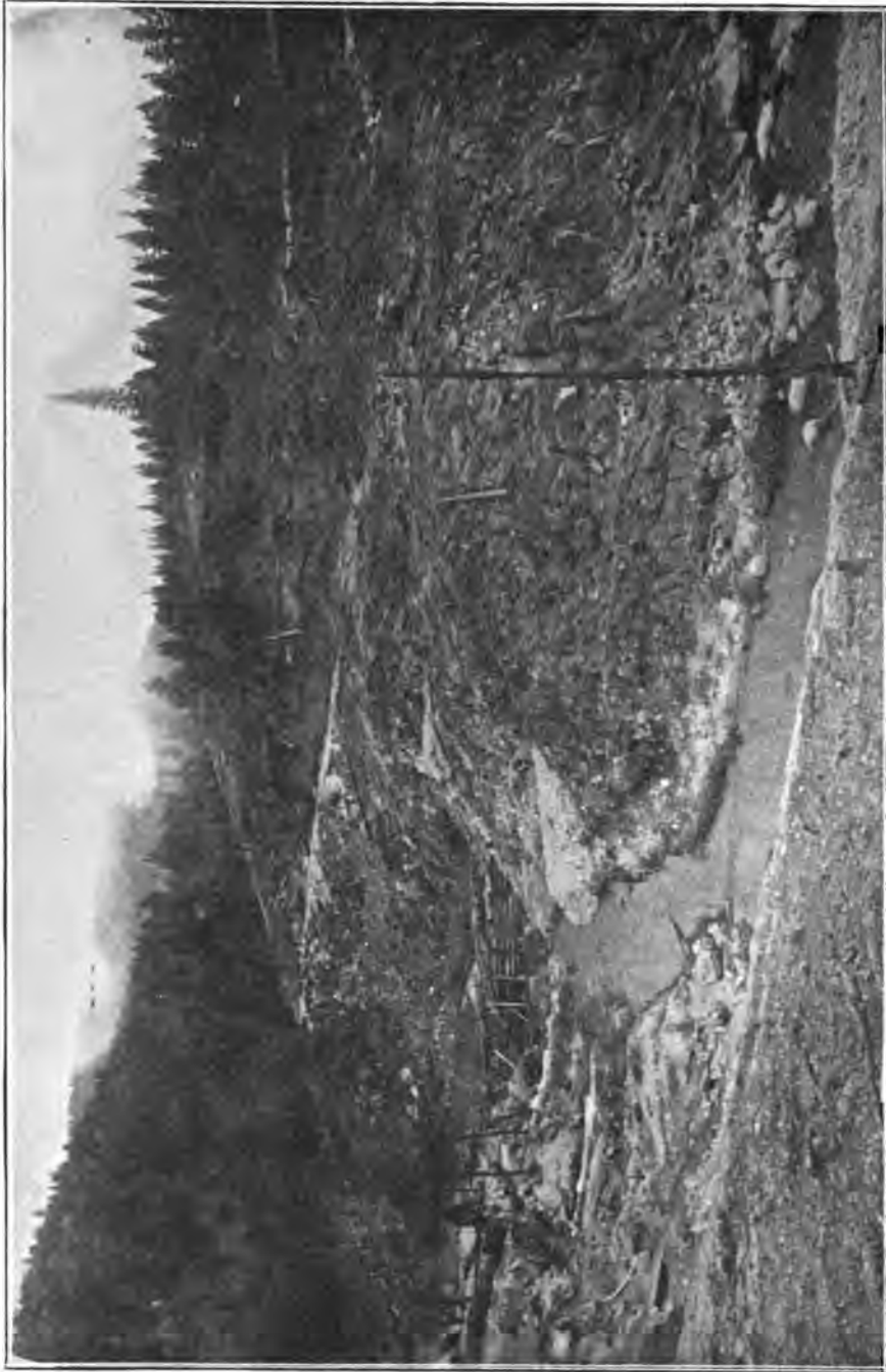
FIG. 488.—VIEW OF LAKE CHRISTINE DAM-SITE, SAN JOAQUIN RIVER, NEAR FRESNO, CALIFORNIA, WHERE A HYDRAULIC-FILL DAM IS IN PROCESS OF CONSTRUCTION.
