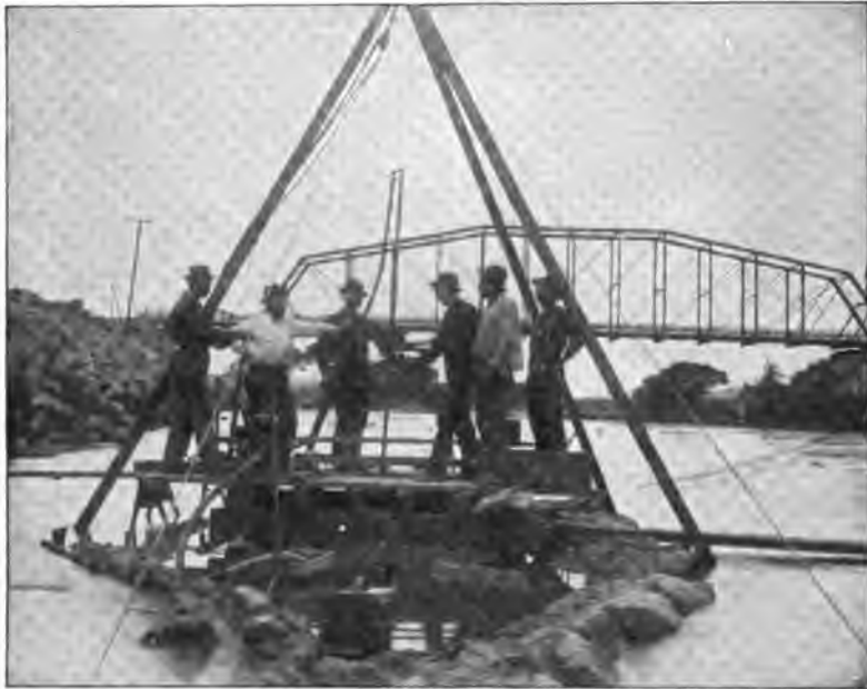
FIG. 153.—BORING APPARATUS, CONSISTING OF PILE-DRIVER AND DIAMOND-CORE DRILL AT WORK. USED FOR TESTING BED-ROCK AT GILA RIVER DAM-SITES, ARIZONA.
