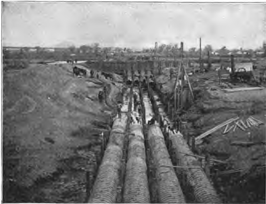
FIG. 170.—WOOD-STAVE PIPES, LAID UNDER BED OF THE RIO GRANDE, FOR SIPHONING CANAL ACROSS THE RIVER, BY RIO GRANDE DAM AND IRRIGATION COMPANY.
