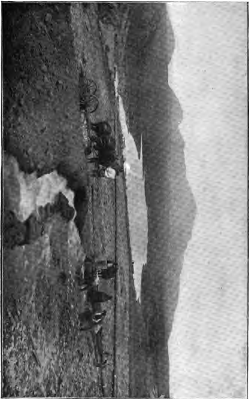
FIG. 484.—LA MEZA (CAL.) DAM IN COURSE OF CONSTRUCTION BY THE HYDRAULIC PROCESS. Showing method of loosening earth to get it in suspension before taking it into carrying conduit. The conduit was built in 30-foot sections, which could be and were frequently taken apart and moved as conditions required.
