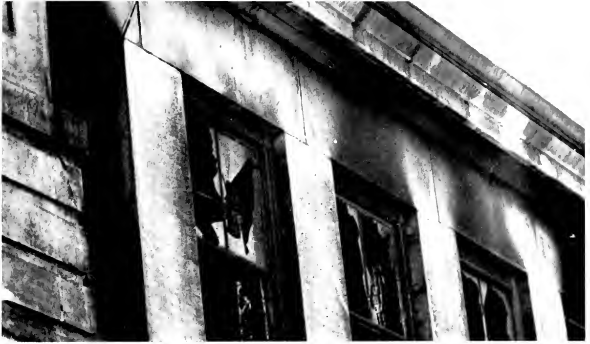
Quincy Building after upper story fire in 1971. photo: Allen McCullough
