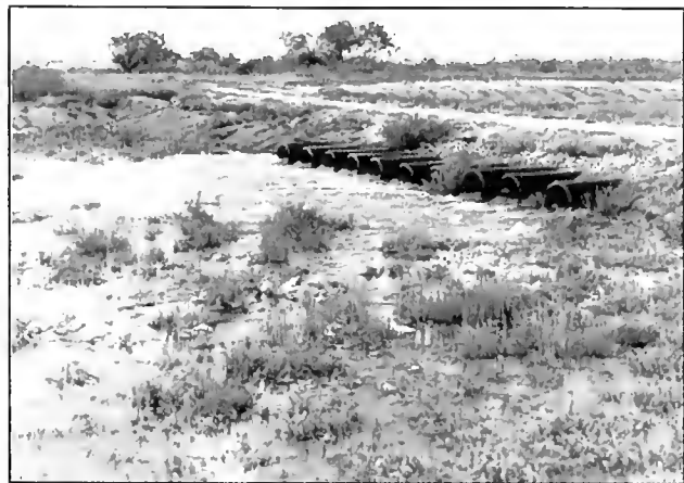
Figure 3-12: Discharge into the tidal flats area through the road crossing at the north end of the Rincon Overflow Channel during Event 16 (June 27, 1997). Each of the 10 corrugated HDPE culverts shown were 24"-diameter. This structure was subsequently washed out during Event 25 (October 1998).
