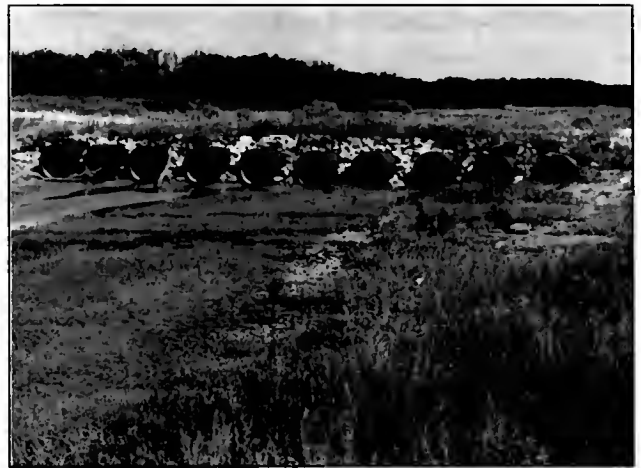
Figure 3-16: The low water crossing at the head of the upper Rincon Bayou channel. The integrity of this structure, although significantly over-topped during Event 25 (October 1998), remained unchanged throughout the demonstration period. Each HDPE culvert was 36"-diameter. The photo was taken on June 1999.
