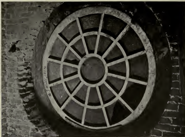
ORIGINAL GABLE WINDOW IN OLD PINE STREET PRESBYTERIAN CHURCH (May be seen by ascending to the loft)
