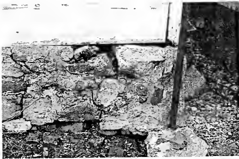
Fig. 2. The character of the masonry is fieldstone with some granite. It is pulling apart at the corners.
