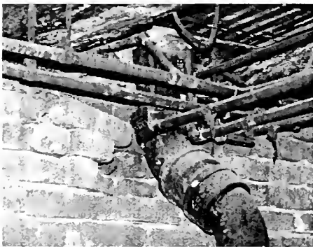
Fig. 4 & 5. Plumber damage in the basement.
