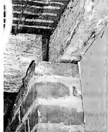
Fig. 3. The beams are pulling free of the sill plate.
