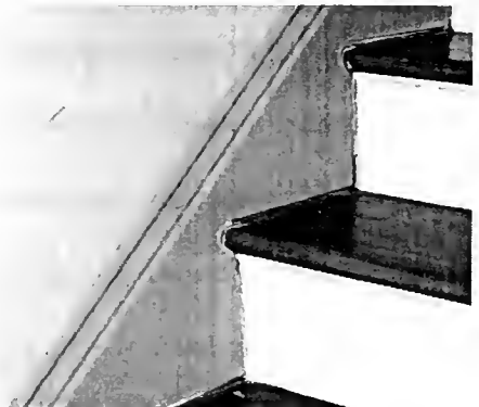
Fig. 12. The gap between the top of the tread and the bottom of the baseboard has been carefully infilled.
