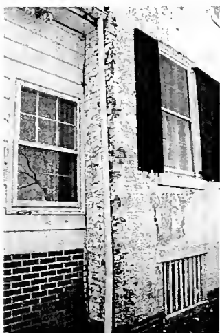
Fig. 15. Paint, stucco, mortar, and brick face are being washed away.
