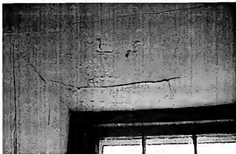
Fig. 9. Water damage above the dormer.
