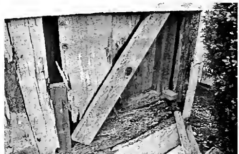
Fig. 1. Exposed rotted framing on the middle building.
