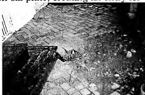
Fig. 10. Something is digging.
