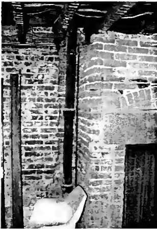
Fig. 13. The moisture from the sewage pipe is rotting the nearby brick.
