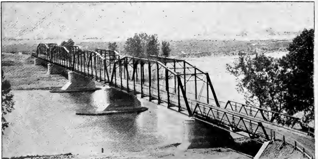
4 Pin Connected Pins 175 Feet Each and 2 Riveted 80 Feet Spans Over Belly River Near Lethbridge.
