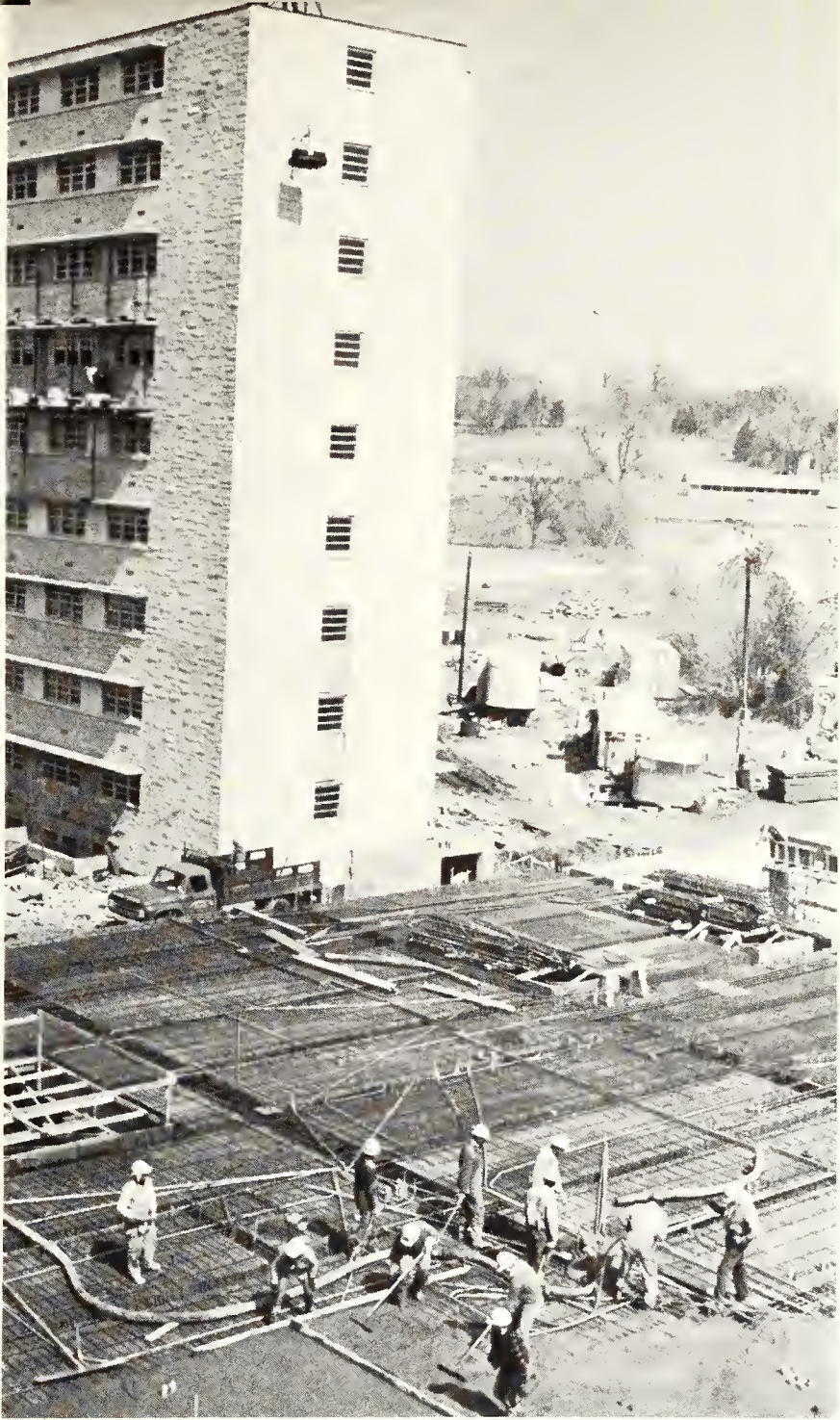
Rising nine stories high, the new women's dormitory overlooks work on the foundation of a food service building.
