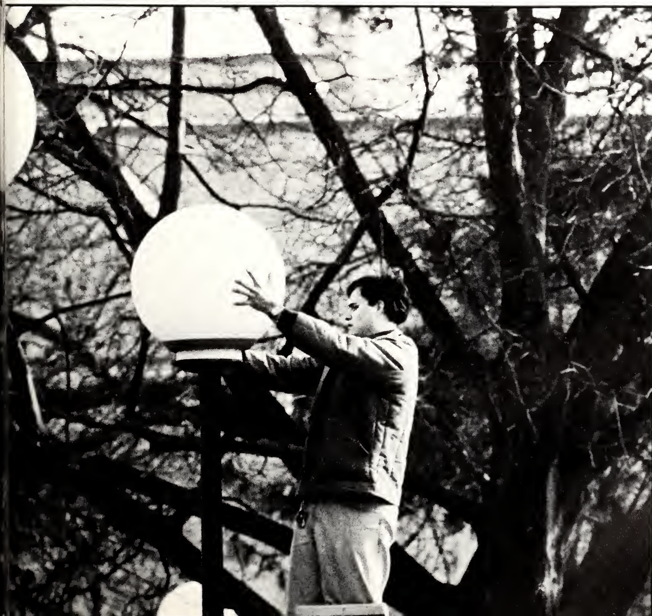
Between Farrell Library and Lafene Student Health Center, David Bradford, junior in mechanical engineering and employee of the Division of Facilities, sets a globe atop a light post after changing the bulb inside. The globe-style lamps replaced China hat-style lamps during mid-campus sidewalk renovations. (Photo by Cary Conover)
