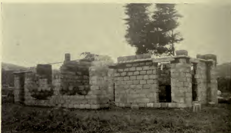
FIG. 28.—Pair of cottages similar to those in Fig. 27, in course of erection.
