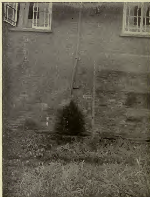
FIG. 16.—Rain-water pipe ending against a wall. The soaking of the wall is well shown. To face page 69.
