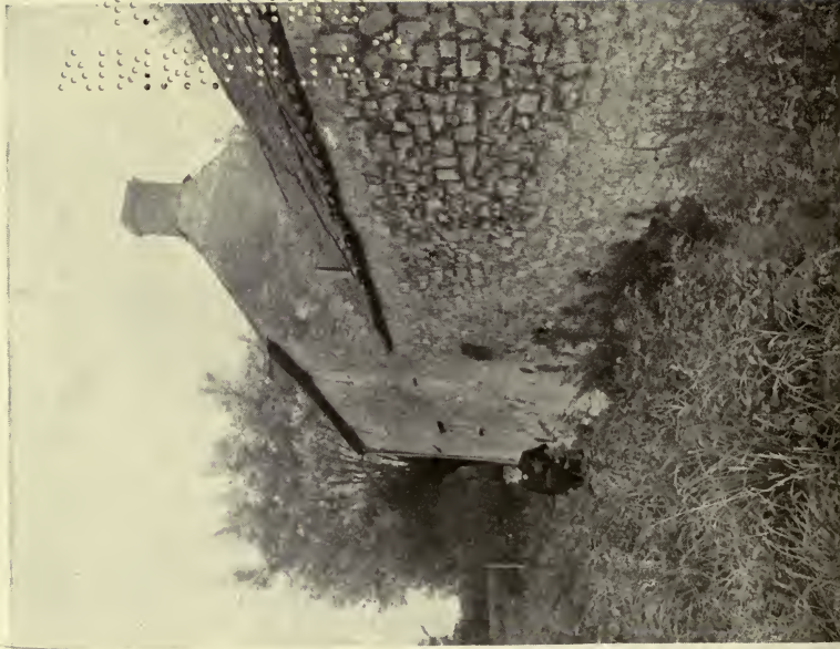
FIG. 14.—Two houses directly abutting against a ditch. At the time the photograph was taken the ditch was dry, but it is full of water for the greater part of the year. This soaks up the walls. The houses have no damp courses or any means of obviating this. The nearest house has neither rain gutters nor through ventilation.
