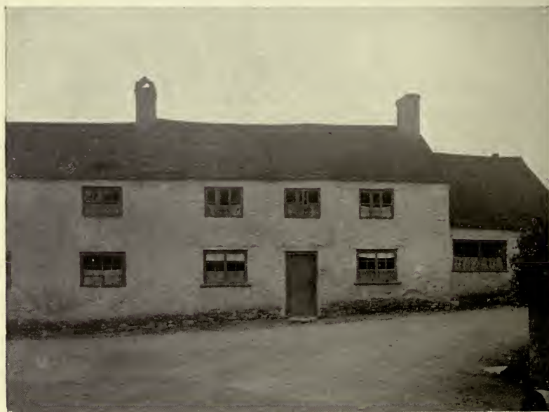
FIG. 12.—Houses without rain gutters, an exceedingly common defect. The rain falls on the ground in front of the houses, and some of it soaks up into the walls. The effect of this damp is very clearly shown by the discolouration and dark fungus growth all along the lower foot or so of the front wall. To face page 65.
