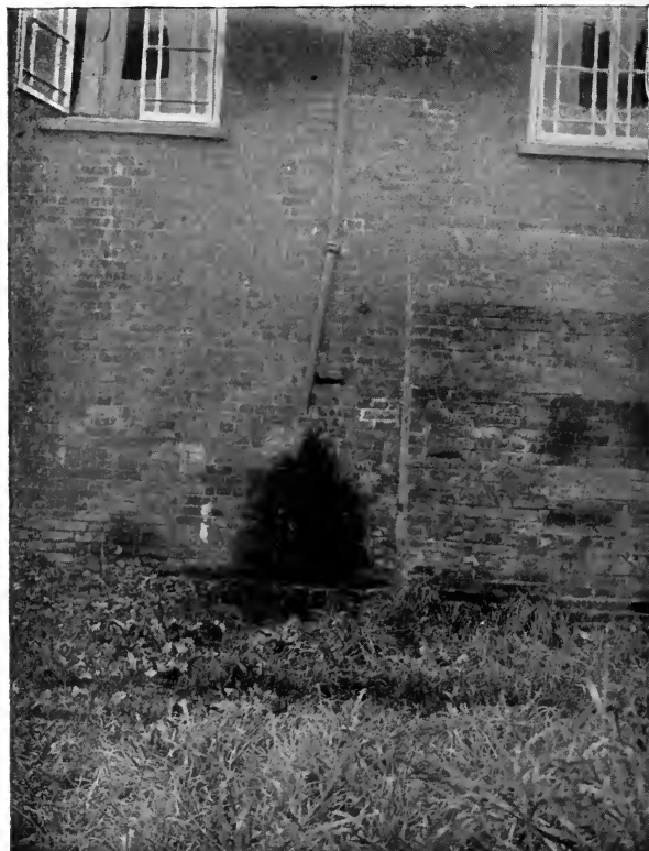
FIG. 16.—Rain-water pipe ending against a wall. The soaking of the wall is well shown. To face page 69.
