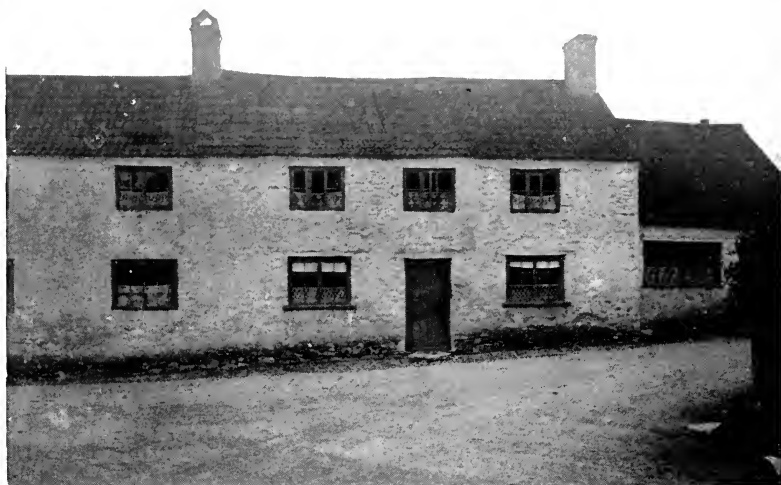
FIG. 12.—Houses without rain gutters, an exceedingly common defect. The rain falls on the ground in front of the houses, and some of it soaks up into the walls. The effect of this damp is very clearly shown by the discolouration and dark fungus growth all along the lower foot or so of the front wall. To face page 65.
