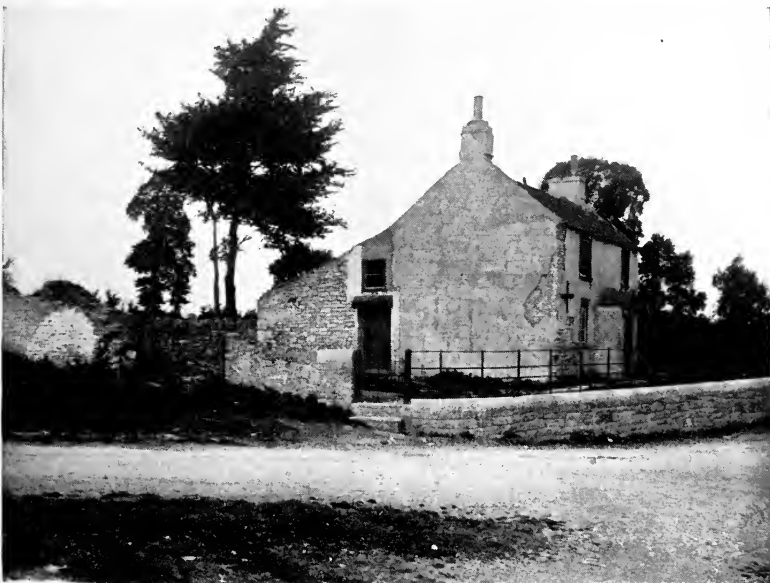
FIG. 25.—An unfit house still occupied, although represented to the Local Authority by their Medical Officer of Health, over two years earlier, as unfit for habitation. The whole house is grossly insanitary.
