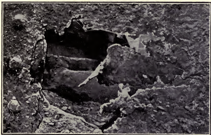
FIG. 48.—Corrosion of a steel plate from the Washington Street railway bridge in Boston.
