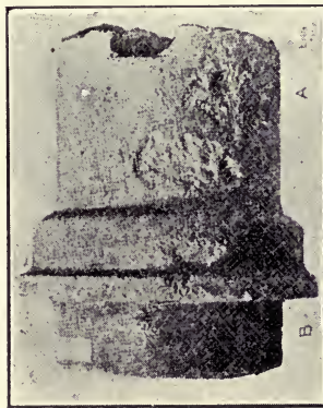
FIG. 76.—Electrolytical pittings on 12-inch cast-iron water-main. (Current flowing from A to B .)
