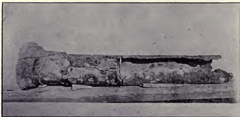
FIG. 80.—Electrolysis of a 6-inch cast-iron pipe at Providence, R. I.
