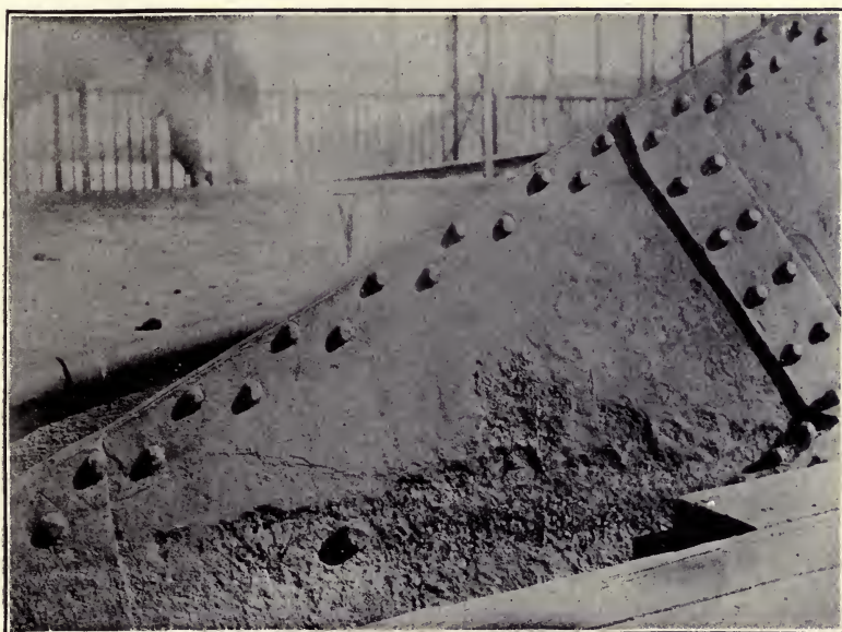
FIG. 81.—Electrolysis of a steel bridge truss.
