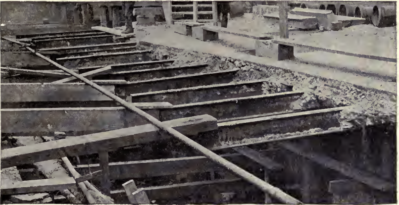
FIG. 38.—Corrosion of sidewalk iron beams.
