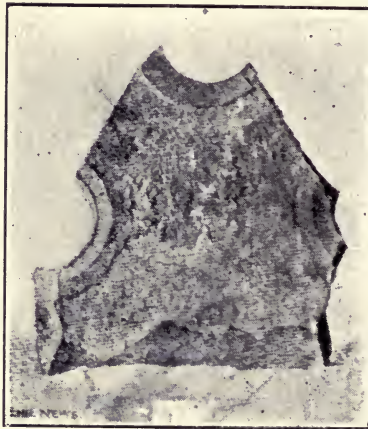
FIG. 73.—Pitting of steel stand-pipe sheet around the rivets.
