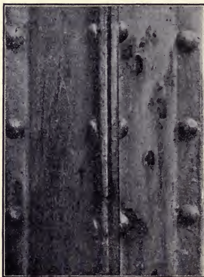
FIG. 36.—Mill-scale corrosion, Phoenix column.
