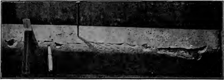
FIG. 82.—Exterior of a pipe injured by electrolysis, Springfield, Ill.
