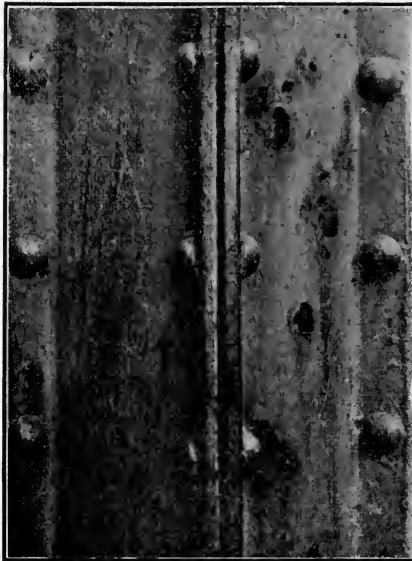
FIG. 36.—Mill-scale corrosion, Phoenix column.
