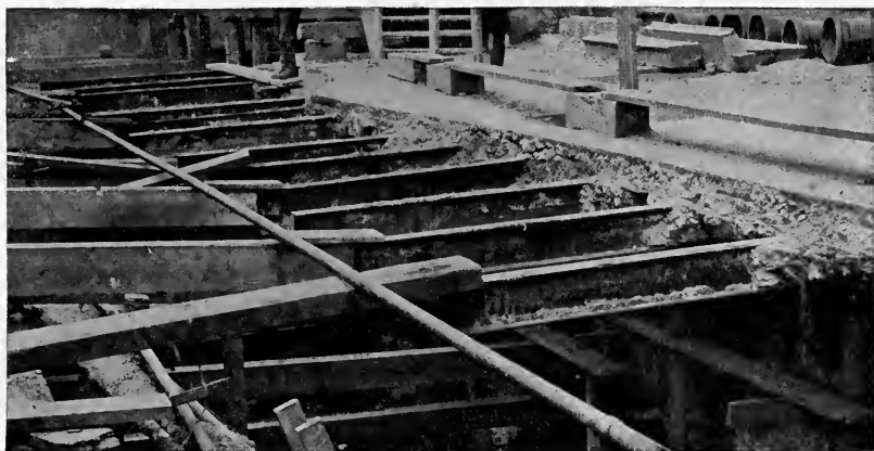
FIG. 38.—Corrosion of sidewalk iron beams.
