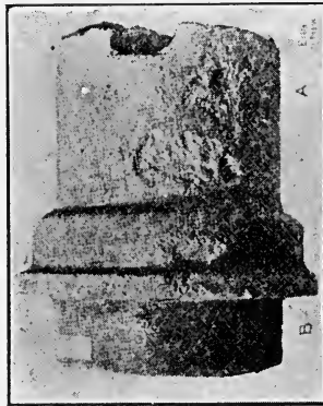
FIG. 76.—Electrolytical pittings on 12-inch cast-iron water-main. (Current flowing from A to B .)
