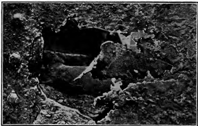
FIG. 48.—Corrosion of a steel plate from the Washington Street railway bridge in Boston.
