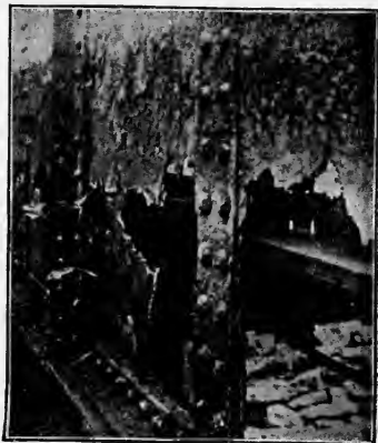
FIG. 47.—Laminated corrosion of a steel-plate girder on the Washington Street railway bridge in Boston.
