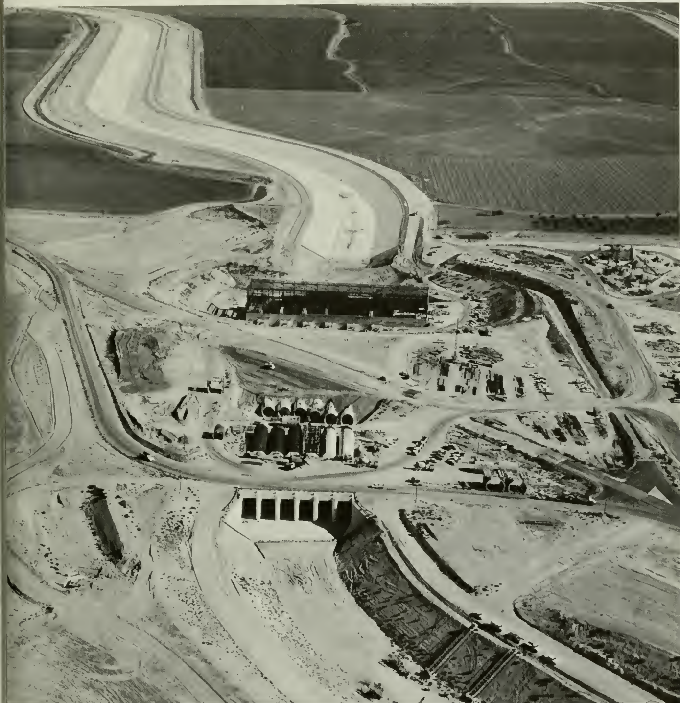
DOS AMIGOS PUMPING PLANT - SAN LUIS CANAL
