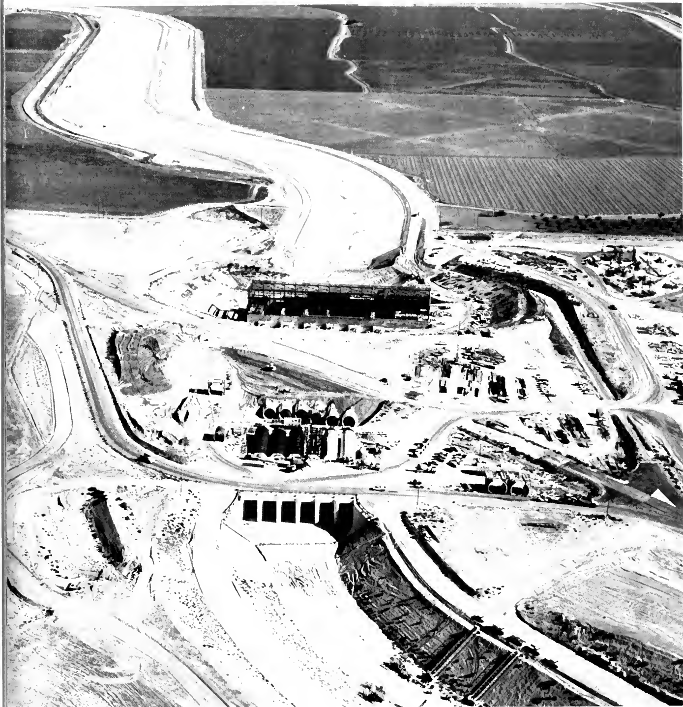
DOS AMIGOS PUMPING PLANT - SAN LUIS CANAL
