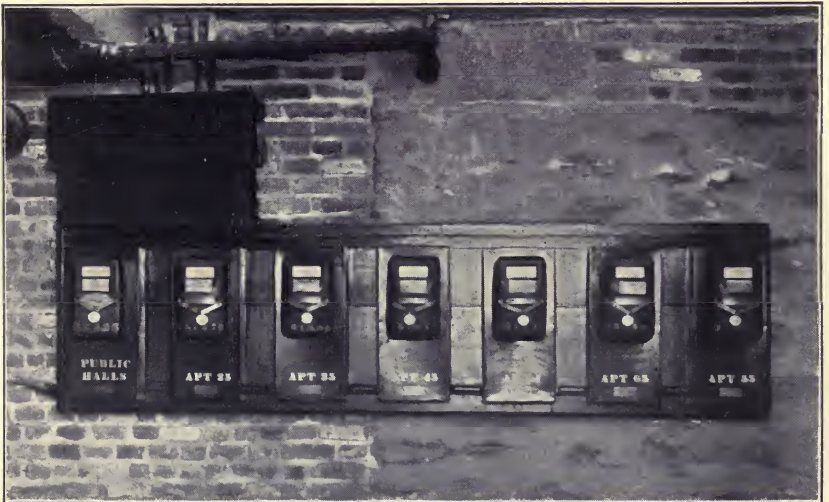
SAFETY DEVICES FOR CONTACT WITH LIVE METAL CONDUCTORS
