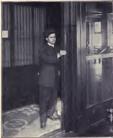
DEVICE FOR ILLUMINATING THRESHOLDS AS ELEVATOR APPROACHES EACH FLOOR AT THE NATIONAL CASH REGISTER COMPANY
