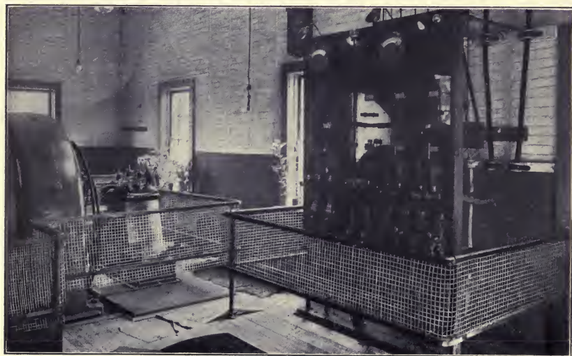
SCREENS AND RAILINGS AROUND DYNAMO AND SWITCHBOARD
