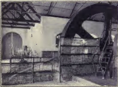
GUARDS AROUND FLY-WHEEL AND CONDENSER PUMP
