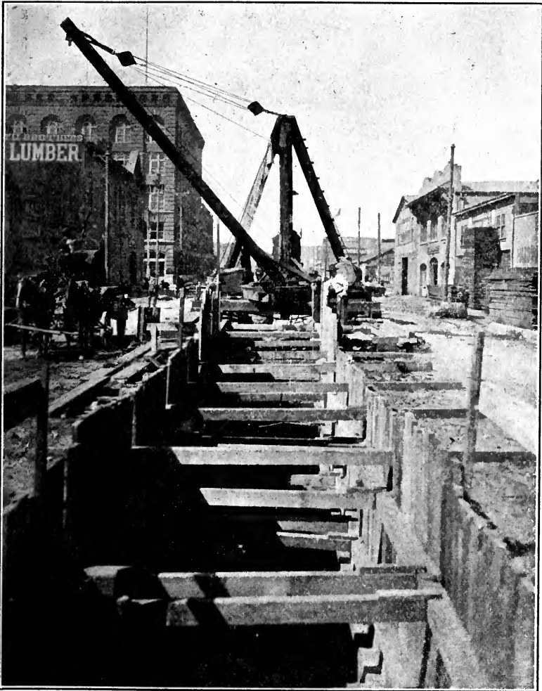
Open trench in Howard Street, near Spear Street, for the construction of a 7-foot 6-inch circular concrete sewer. All material excavated from the trench was at once removed in wagons and the street kept open for traffic.
