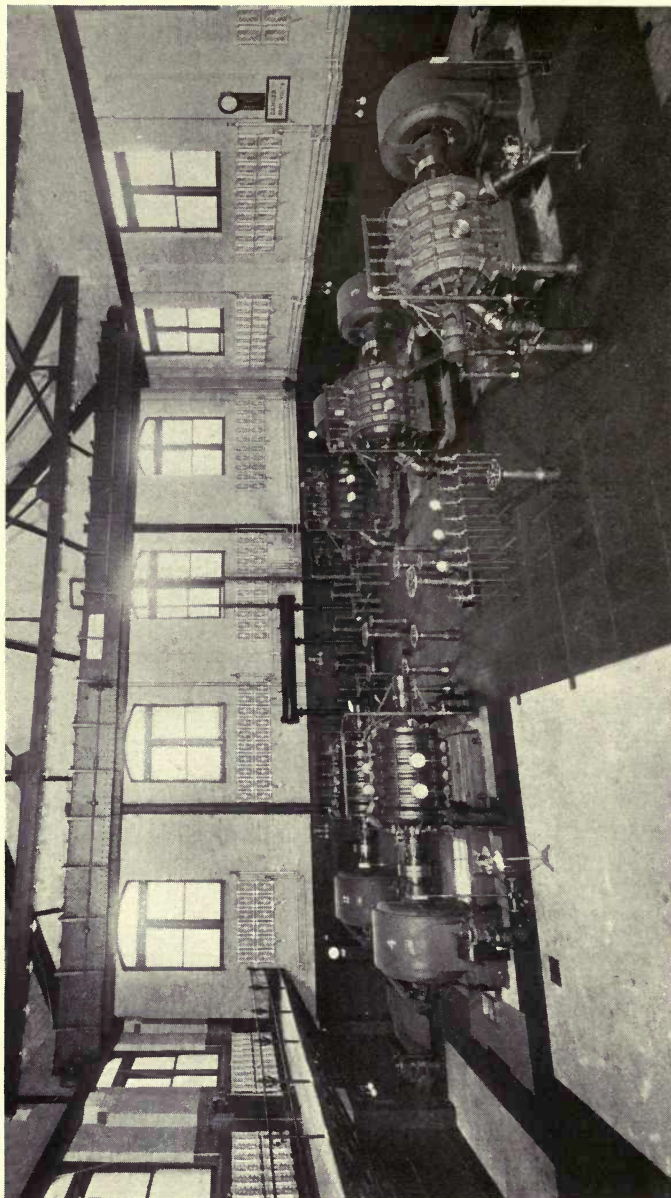
NEW YORK CITY, BOROUGH OF BROOKLYN High Pressure Fire Service Station
