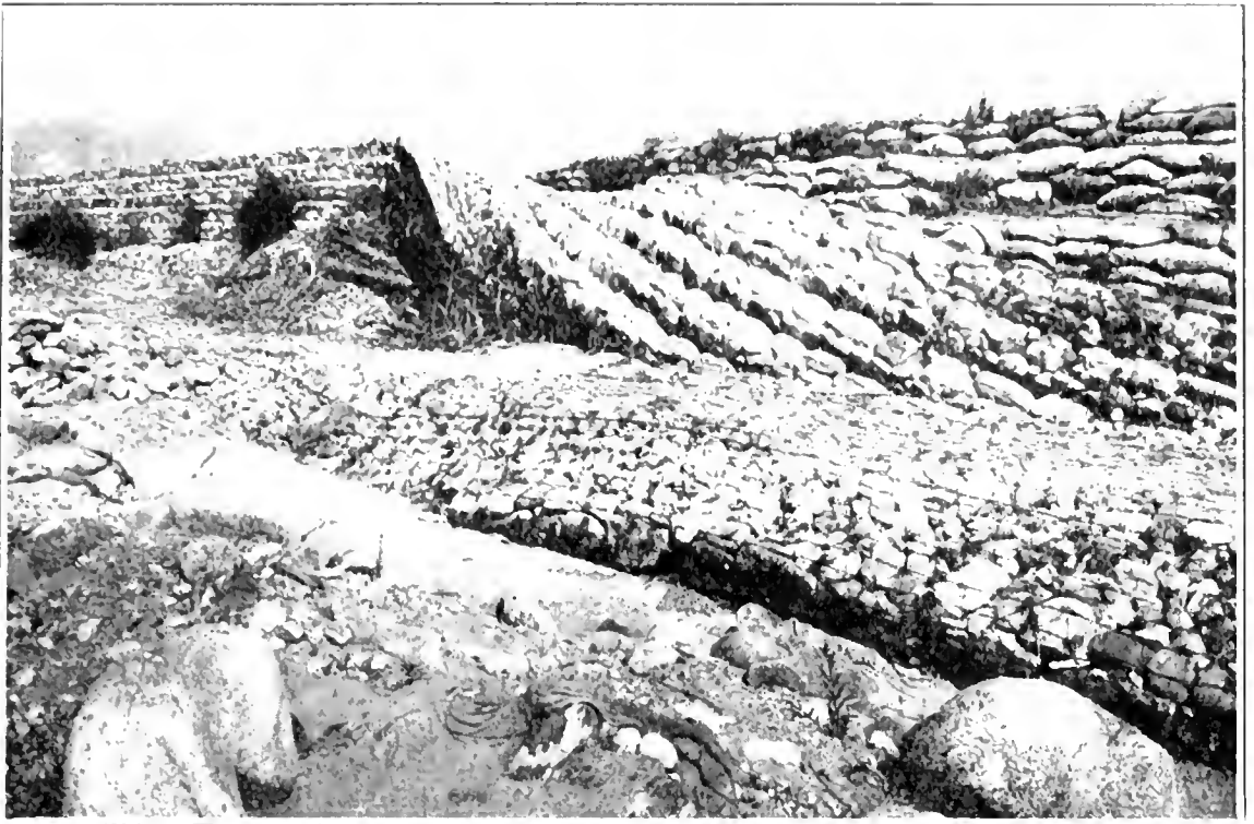
FIG. 13—Channel Control. Rock wall mattress overturned on San Gabriel River north of Foothill Boulevard.
