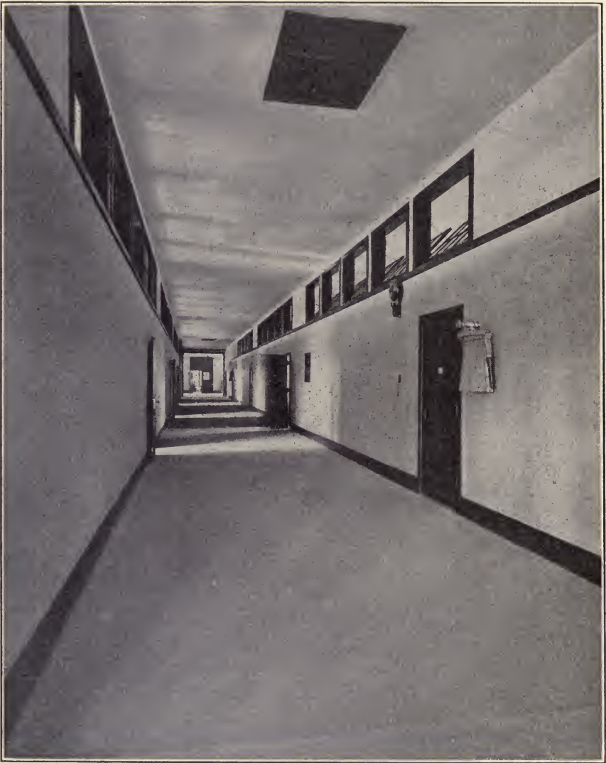
A modern corridor, showing arrangement of transoms opening from classrooms. Note ventilation, fire gong and hose reels.
