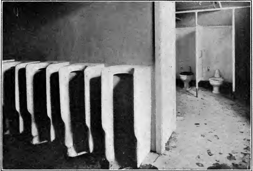
Modern up-to-date plumbing. Vitreous china urinals and toilets with utility chamber.
