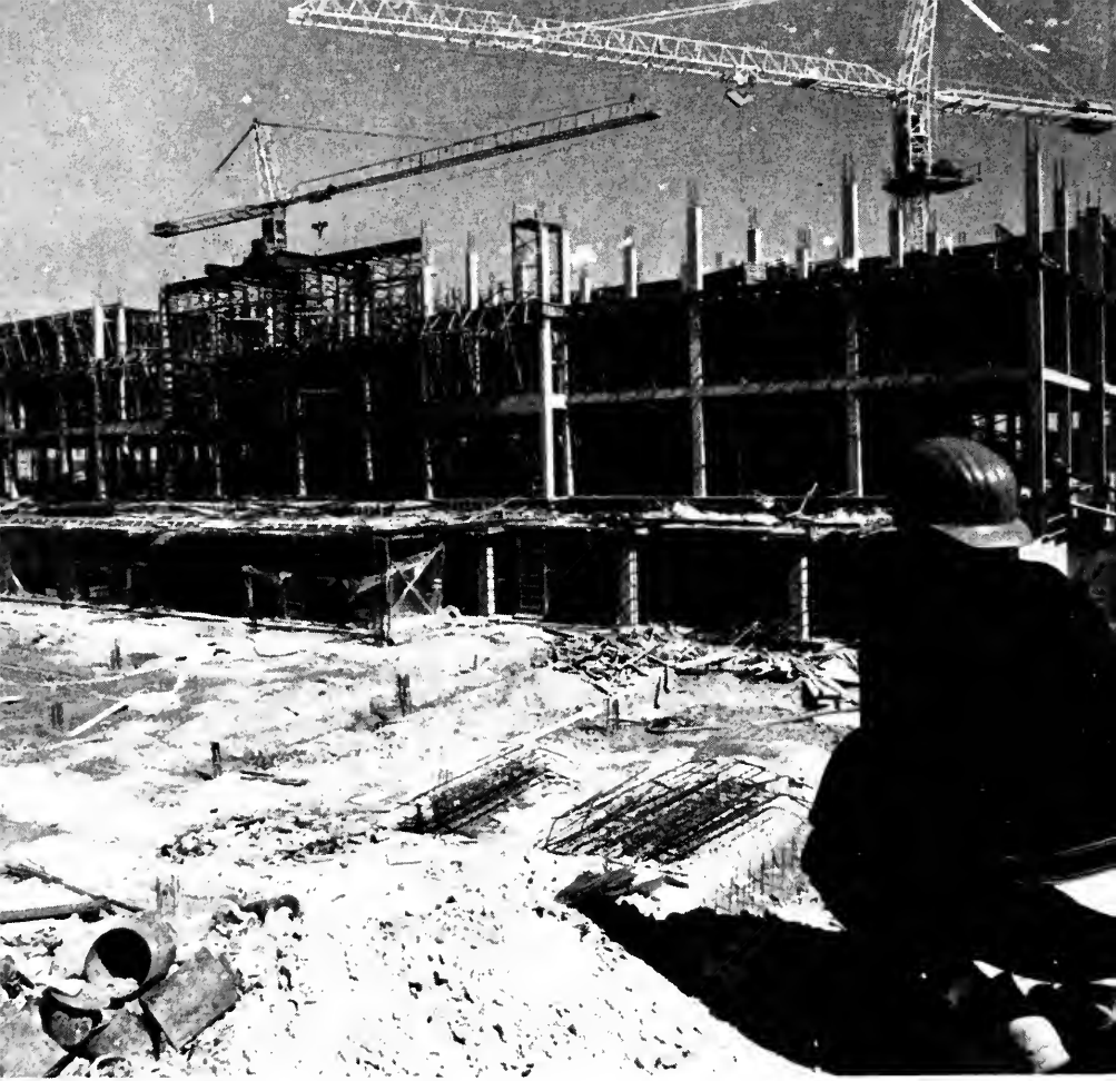
Construction continues on the new undergraduate library and new home of the School of Library and Information Services, scheduled for completion in November 1972
