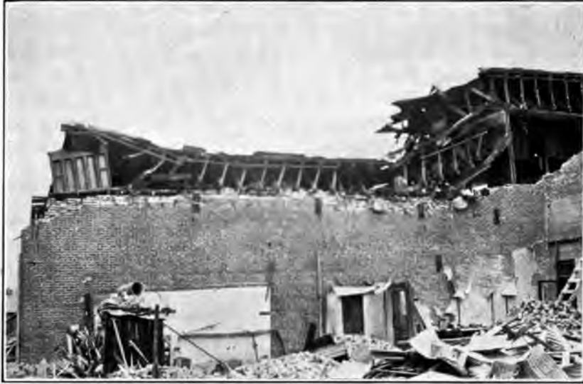
FIG. 9. MASONIC HALL AT SAN JACINTO, CALIFORNIA, wrecked in the Earthquake of April 21, 1918. Note the piano under the roof at the left. Brick buildings can not withstand severe earthquakes. (Photograph by Homer Hamlin.)
