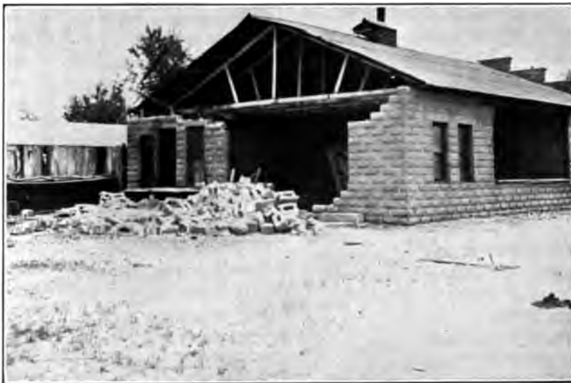
FIG. 16. A CONCRETE-BLOCK BUILDING WRECKED BY AN EARTHQUAKE. Experience has shown that reinforced concrete, steel-frame and wooden buildings will stand through severe earthquakes, whereas brick, concrete-block and adobe buildings are easily destroyed. (Photograph by Homer Hamlin.)
