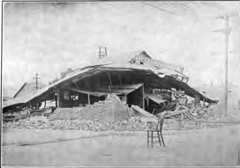
FIG. 2. AN EXAMPLE OF THE DAMAGE SUSTAINED BY BRICK BUILDINGS IN AN EARTHQUAKE. The reinforced concrete building shown in the right background was comparatively unharmed. (Photograph by S. D. Townley.)
