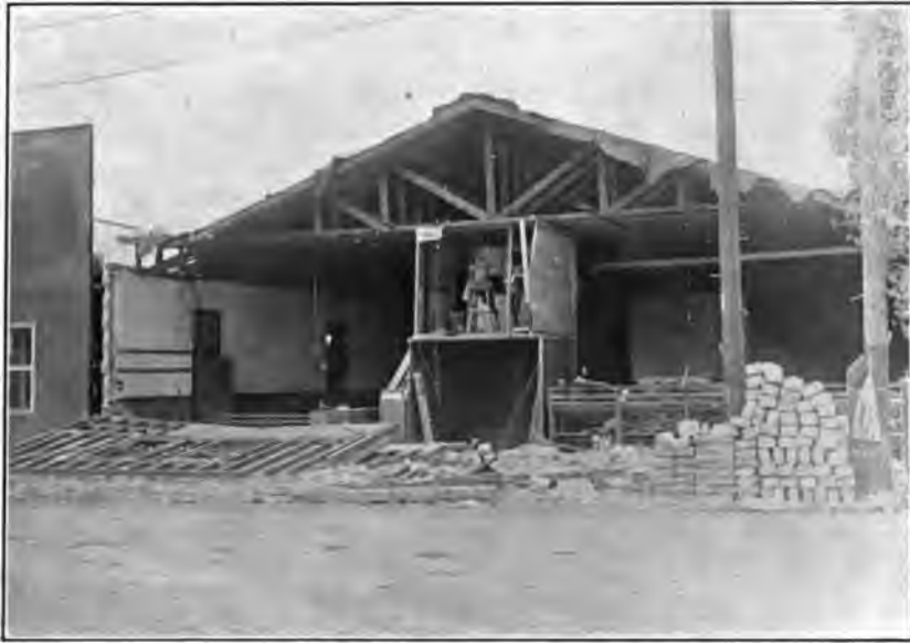
FIG. 1. A MOVING-PICTURE THEATER AT SAN JACINTO, CALIFORNIA, AFTER ITS FRONT WALL HAD FALLEN TO THE STREET DURING A RECENT EARTHQUAKE. The concrete-block type of construction is dangerous in a region of high seismicity. (Photograph by S. D. Townley.)
