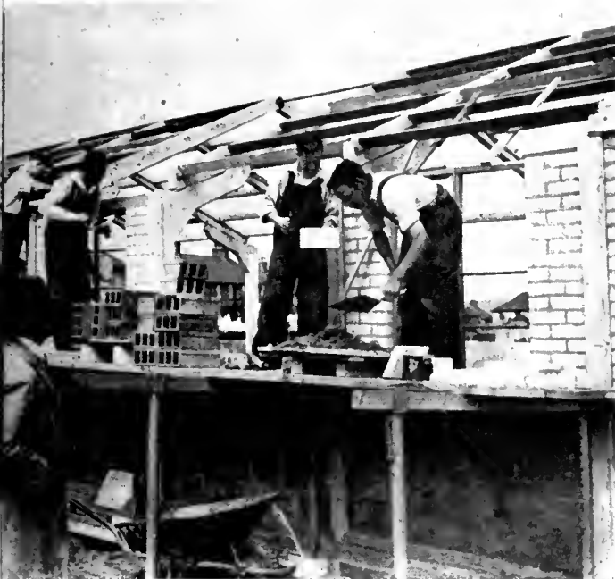
Members of the youngest building team in Britain working on a nursery school. (See "New Builders")
