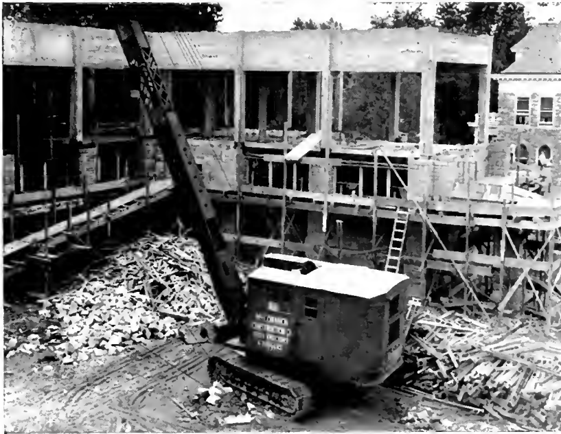
While the girders were being put in place, construction was delayed by a general strike. This picture was taken some-time after operations were resumed.
