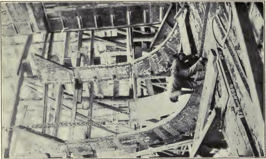
An Erecting Gang at Work on the Hull of a Steel Ship
