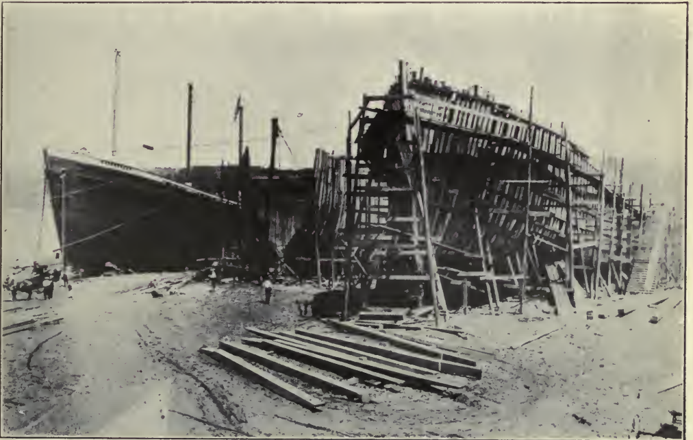
At the left, ship ready for launching; at the right, ship fully framed, ready for planking.
