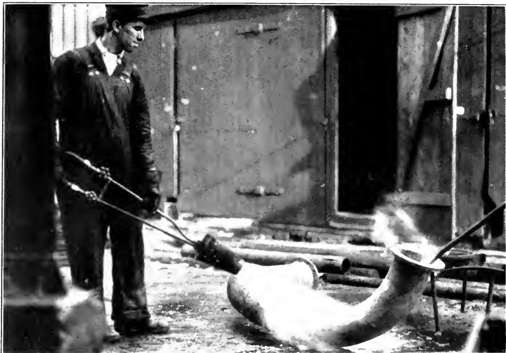
Heating Pipe From the Copper Shop With An Oil Blast
