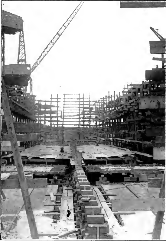
Ship carpenters have erected the scaffolding about the "berth" and laid the keel blocks down the center.
