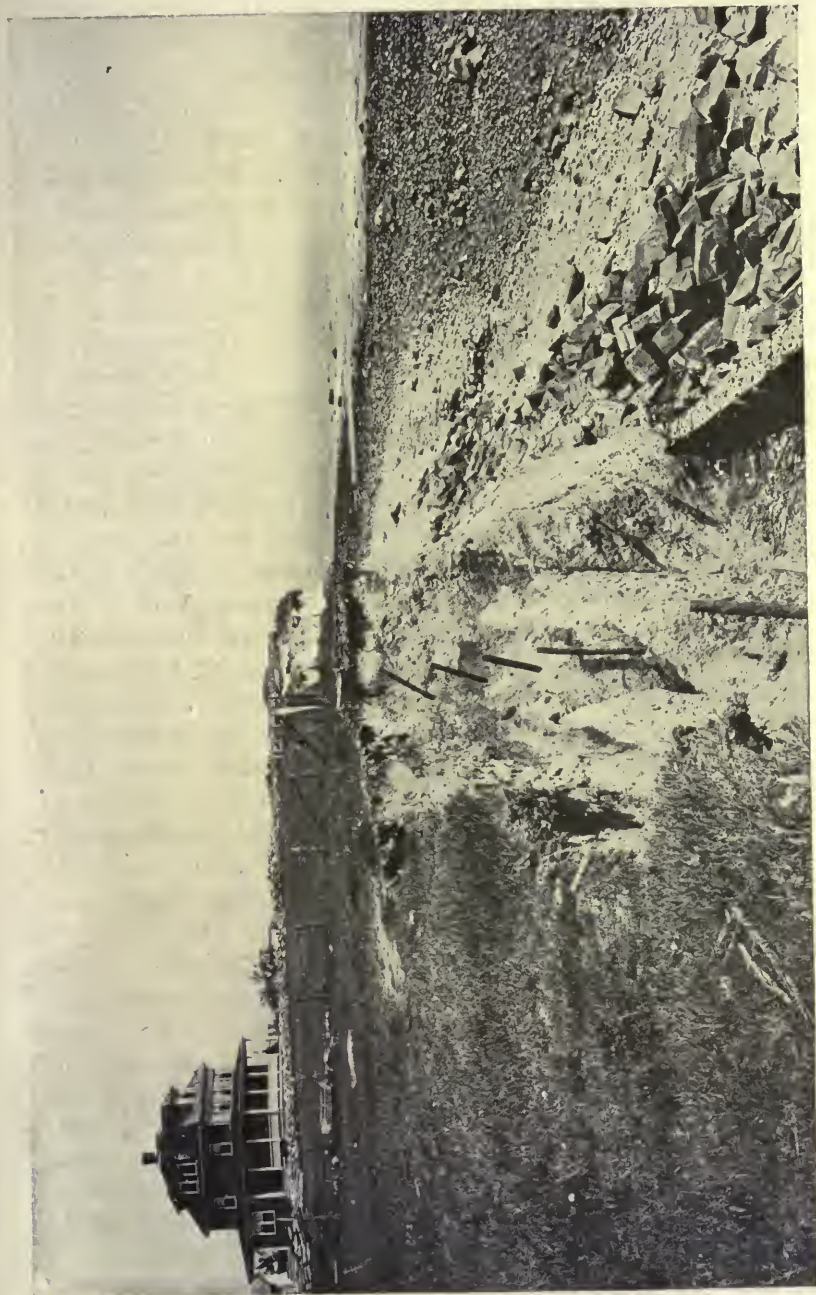
Wire fence undermined by wave attack and left hanging in mid-air. The road in front of the house has been completely cut away. Third Cliff, Scituate, Massachusetts.
