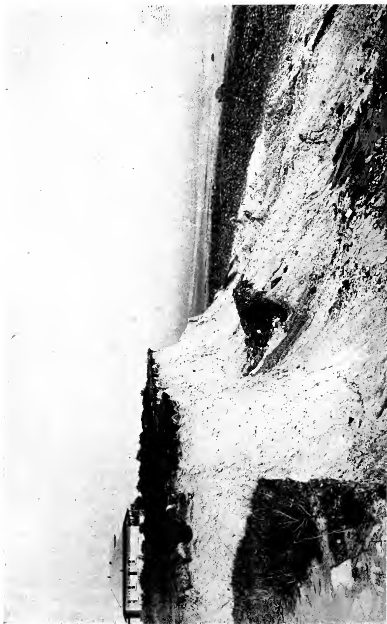
Third Cliff near Scituate, Massachusetts, showing small landslide due to wave erosion of cliff base.
