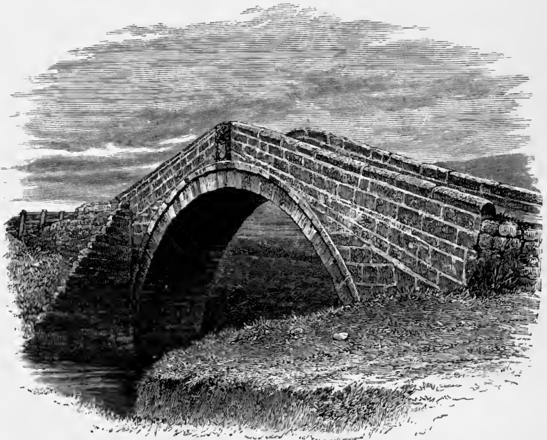
BRIDGE OVER THE ESK AT DANBY IN CLEVELAND. Late in the Fourteenth Century.
