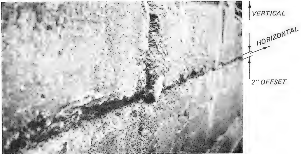
Figure 34. Photograph of offset (approx 2 in.) between concrete caissons in Quebec Harbor, Canada
