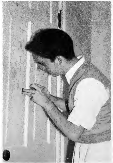
CONSTRUCTIVE HELL WEEK Pledge John Davis '46, executes skilled craftsmanship in constructive house repairs prior to initiation.
