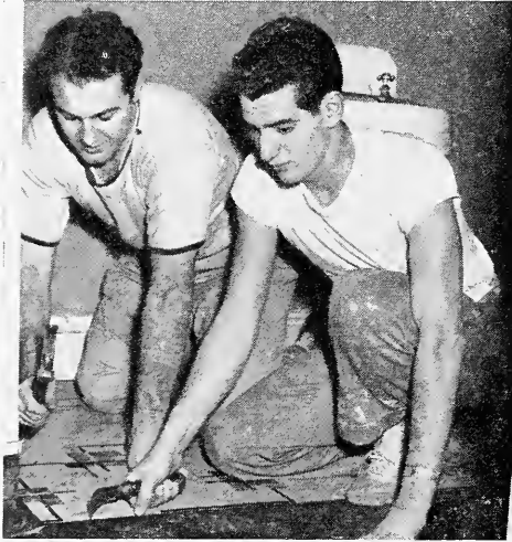
Ferd Cardano and Ed Howard of Lambda Chapter make some needed repairs during Work Week.
