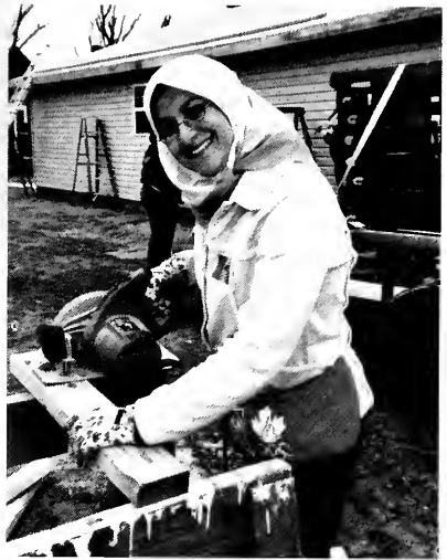
Workin' Hard: Kaleh Karim saws a board that will be used to build the house.
