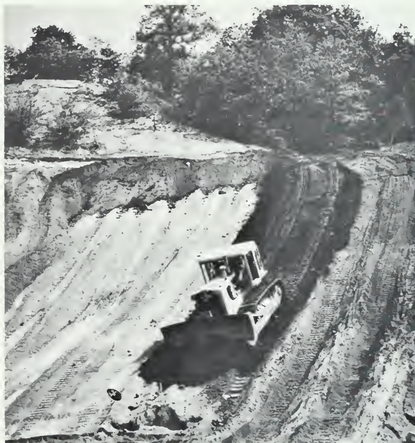
Figure 75 — Both land form design and planting arrangements provide needed transition screens for the operating site
