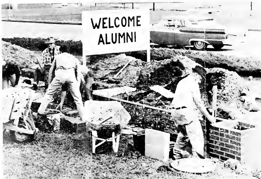
A temporary welcome sign was erected on the site of the new entrance sign, presently under construction. The new sign is a gift of the Alumni Association.
