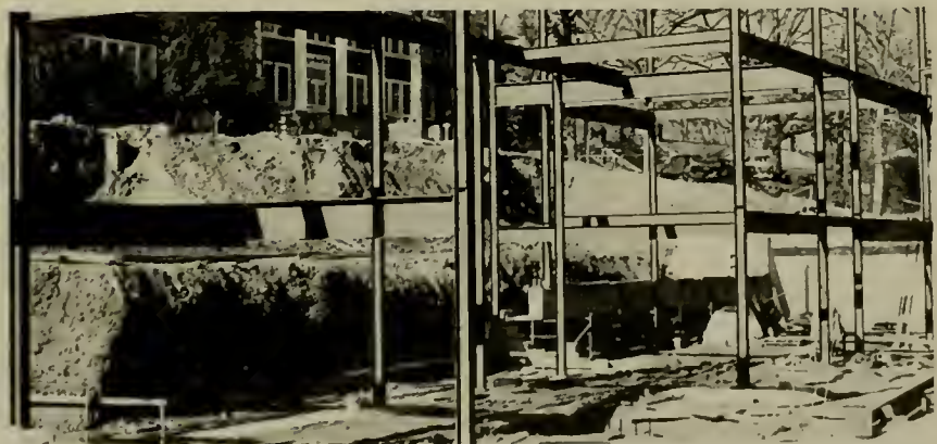
This picture shows the progress on the new cafeteria building which is being erected on the site of the former cafeteria just back of Wright Hall. The old tabernacle houses the food service department until the new one is completed.
