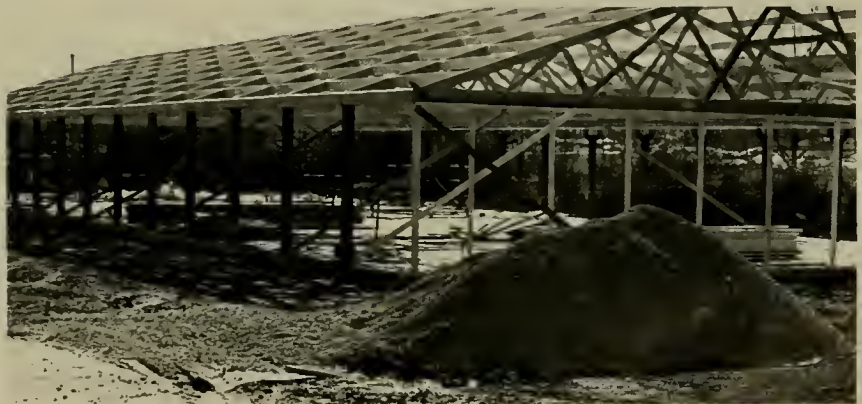
The new greenhouse in which hydroponic tomatoes hopefully will be produced commercially.
