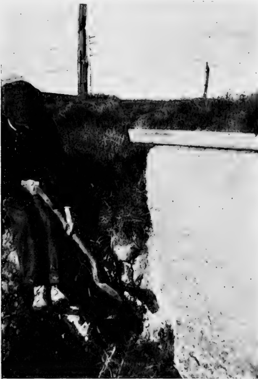
FIG. 24. — POORLY MADE CEMENT THAT IS BEING CRUMBLING BY ALKALI.
