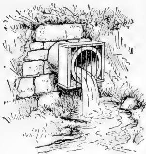
WATER ISSUING FROM AN UNDERGROUND DRAIN. 1
