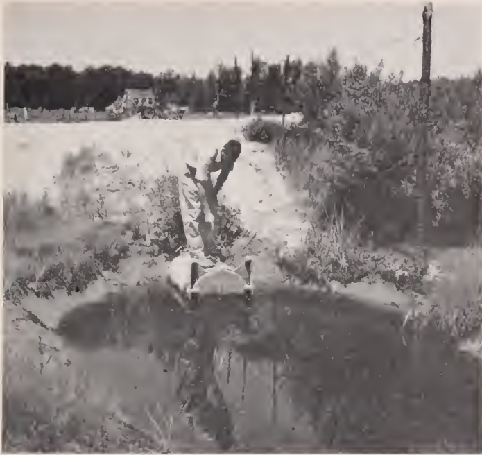
Figure 1.—Tide gate through a dike. The gate prevents water from high tides entering the pipe and flooding areas of Othello silt loam, low. At low tide, the gate opens and excess water is released.
