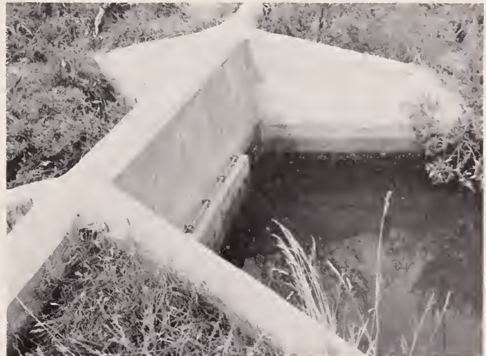
Figure 6.—Concrete structure and tide gate used to control tidal waters on an area of wetland so that adjoining areas will not be flooded by salt water.
