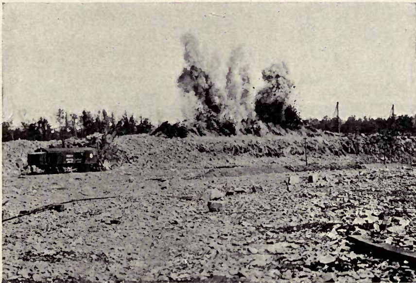
MODERN LIMESTONE QUARRYING AT THE SYRACUSE QUARRIES. 2,000 POUNDS OF DYNAMITE WERE USED IN THIS SHOT.
