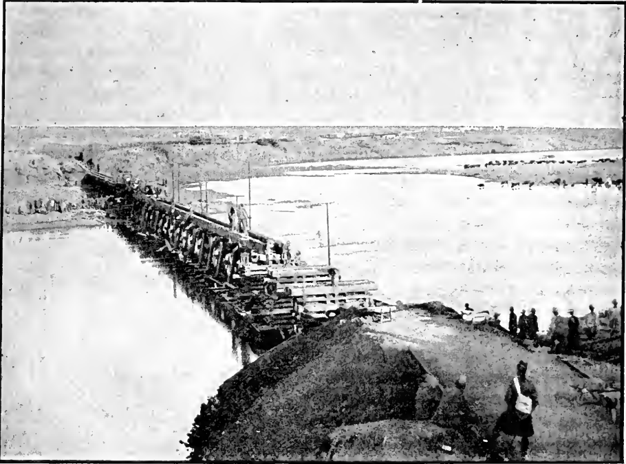
VAAL RIVER DEVIATION BRIDGE AT VEREENING, NEARLY COMPLETED. (Photo by W. H. Gill, London.)
