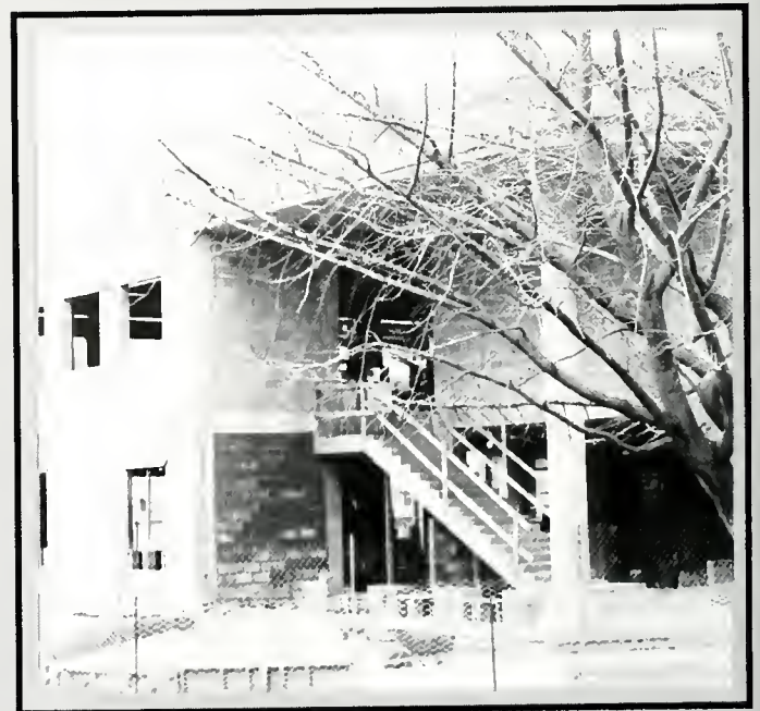
Even at this point in the construction, the annex's contemporary architecture is noticeable.
