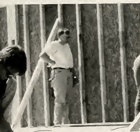
HAMMERS AND NAILS Lay Ryan hammers 2x4's together during a Habitat for Humanity workday. Many students give their time for this cause.
