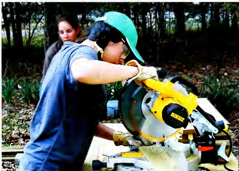
Maria Caycedo '10 working in Greensboro, Alabama. This interim worked with HERO Housing Resource Center to build a wheelchair ramp for a local family during the month of January.
