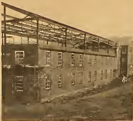
The new wing going onto the Women's Residence Hall will be ready for occupancy in September of 1964. At this time, all structural steel is in place and the wing is ready for the floors and roof.
