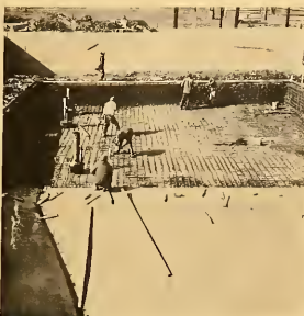
Cox Engineering Co. of Birmingham, Ala. is making rapid progress on the new swimming pool being built in connection with the new P.E. Center.
