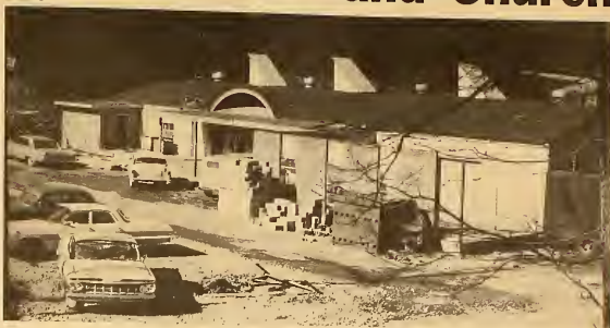
The College Laundry is getting a face lifting that will result in a new office and customer counter space.
