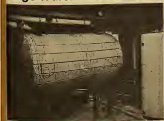
New 500-gallon holding tank installed in Talge Hall recently solves the hot water problem by supplementing the older heaters (right) and adding storage area.
