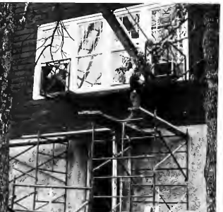
B and G workmen assemble the fire escape recently installed on the north end of Lynn Wood Hall.
