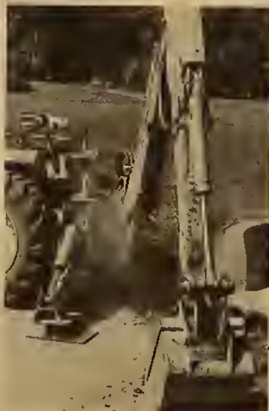
Machine scoops earth away to bare steam rupture.
