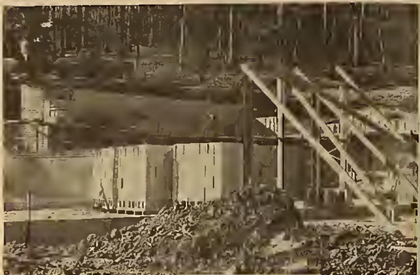
The old, abandoned Collegedale Academy building has been razed to make way for the new home economics center, now under construction.
