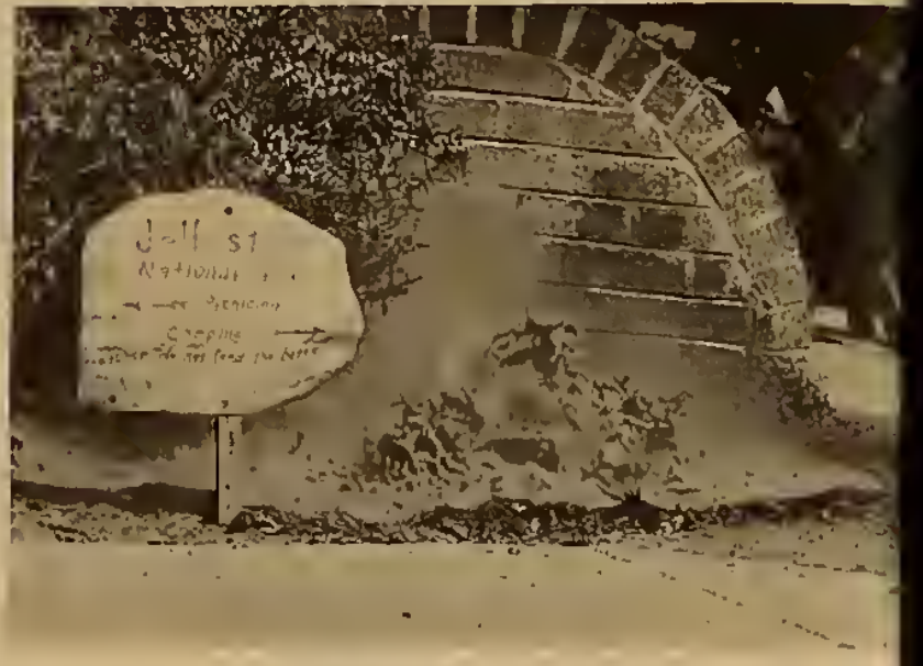
Steam pipe ruptures five feet under ground.
